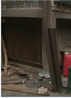
Fig. 5 Buckling of a timber-framed house support column (containing geometric nonlinearity due to the continuous upper structural gravity) [Video #1]
