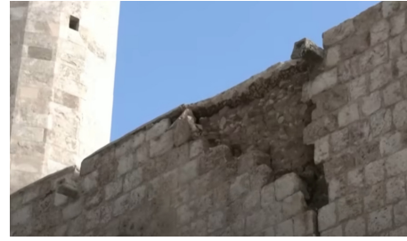
Fig. 3 Spalling of the brick shear walls (containing the material nonlinearity) [Video #2]
