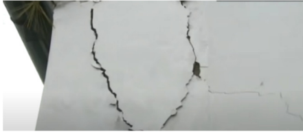
Fig. 1 Cracks in the wall due to the seismic wave (only linear response is generated because the crack is static) [Video #1]
