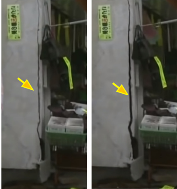
Fig. 2 Cracks in the wall that open and close under the action of the earthquake (containing nonlinear response due to the opening and closing of the cracks) [Video #1]
