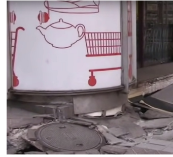
Fig. 7 Damages of the support column (containing boundary-condition nonlinearity. At the same time, the change of boundary conditions will lead to the redistribution of the internal forces of the upper structure. Therefore, it will also cause nonlinear behavior in the upper structure) [Video #5]
