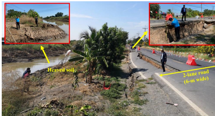
Fig. 3 The Failure of Roadways near the Canal Side at AY. 1043
