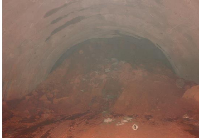
Fig. 7 Collapse situation of the right tunnel
