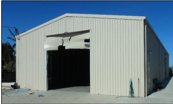
(b) Large opening in the middle of the gable end wall
