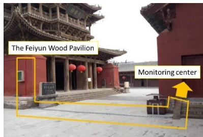
Fig. 18 Electric cable transmission
