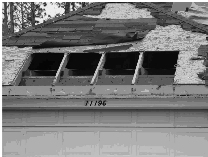
Fig. 3 Loss of roof panel picture from hurricane Katrina (van de Lindt and Dao 2008)
