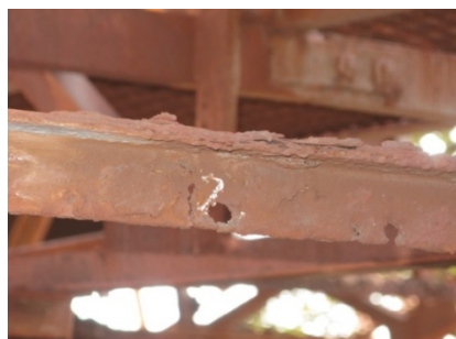
Fig. 21 A corroded part of member 2
