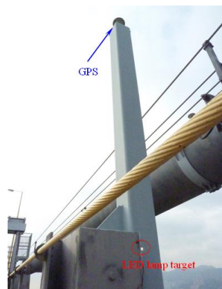
Fig. 14 LED lamp target and GPS receiver installed on Tsing Ma Bridge
