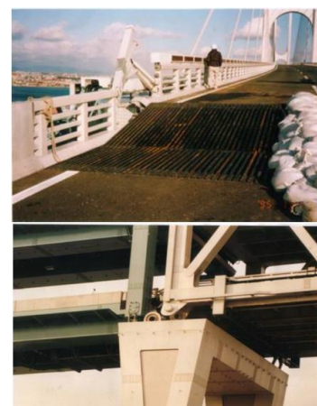
(b) Damage at end-bearing
