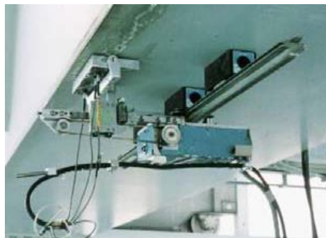
Fig. 25 Automated Ultrasonic Testing system for fatigue crack inspection on HSBE bridge girder. (Okuda et al. 2010)
