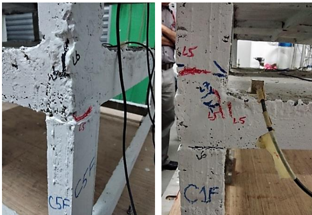
Fig. 19 (b) Flexural horizontal and vertical cracks at a beam-column joint in storey 1
