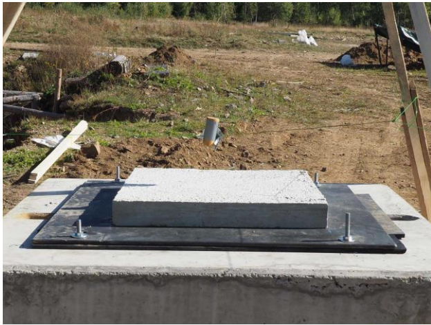
Fig. 7 Incorrectly placed charge
