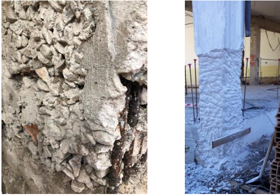
Fig. 6 a) Low quality concrete in a perimeter column; b) Total absence of stirrups in a corner column
