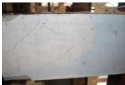
(a) cracking at beam end
