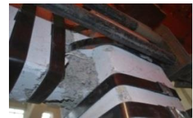
(c) concrete collapse
