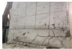
(b) cracking at column
