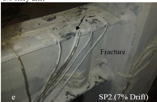
(e) Fracture in the left beam at 7% story drift
