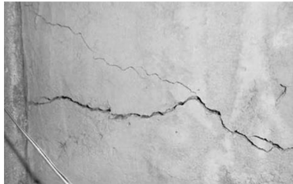
(a) Transverse cracking on the bottom of the concrete slab
