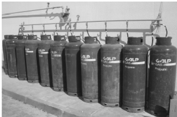
Fig. 6 Battery of gas reservoirs
