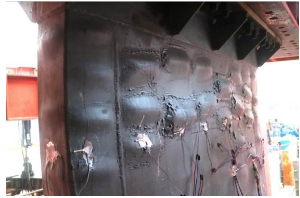
(b) Severe buckling on side S
