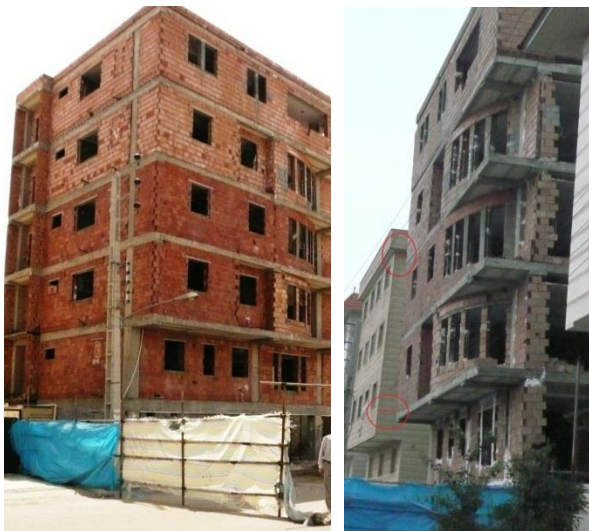
Fig. 3 Rotation of building caused by foundation shear punch
