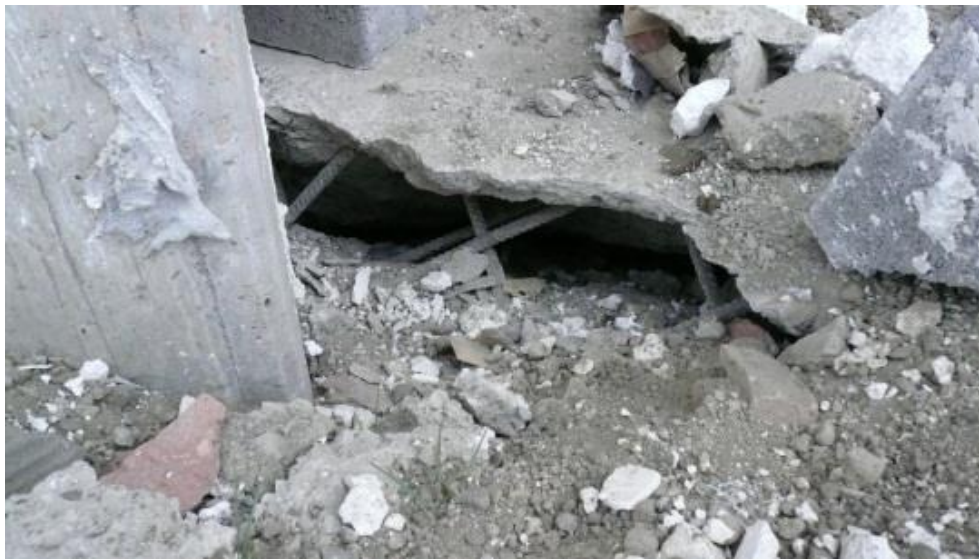
Fig. 20 Foundation shear punch under column B-2 in constructed building
