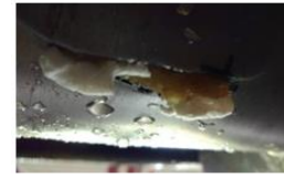
(c) Pipe with corrosion defect and repaired with thermosetting liner
