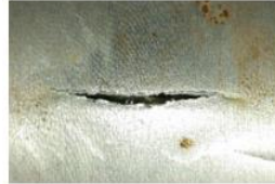
(b) Pipe with corrosion defect
