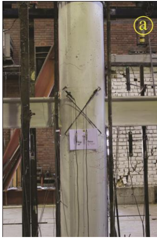
(a) Cracks on the column at about 1.5% storey drift
