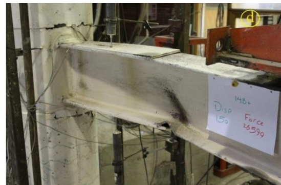
(d) Buckling of beam web at about 5% storey drift
