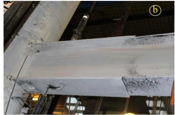
(b) Beam yielded at about 4% storey drift
