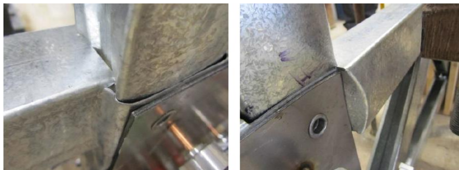
Fig. 17 Sideways buckling failure of the compression chord
