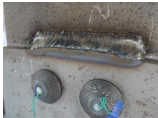
(b) Combination joint (crack angle > 45°)
