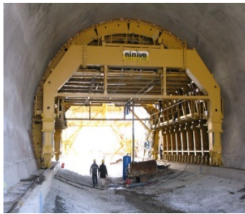
Fig. 5 Examples of tunnel equipment for supporting unfinished tunnels
