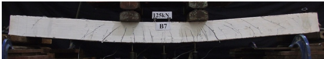
(a) Flexural failure in B9
