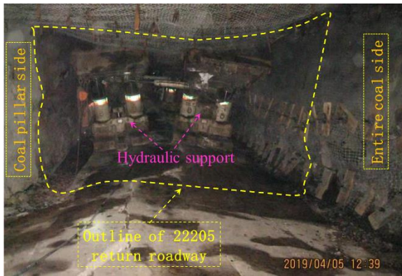
Fig. 21 Advance hydraulic support
