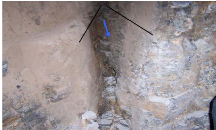
Fig. 16 Wedge failure observed in exploratory drift at P50
