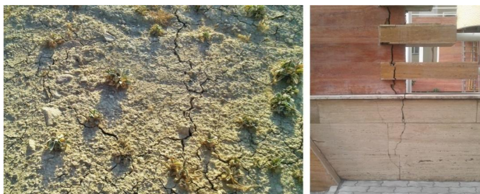
Fig. 4 Cracking walls in residential buildings located in Vali-Asr area of Tabriz (right) and desiccation cracks in the marls due to shrinkage (left)
