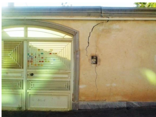
Fig. 3 Cracking on walls of residential buildings due to marls swelling phenomena in the Vali-Asr area
