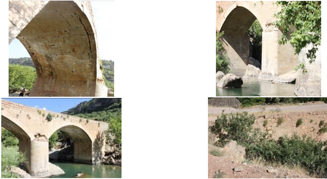
Fig. 2 Deteriorative and hazardous conditions of the bridge
