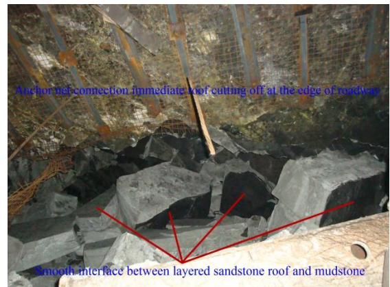
Fig. 6 Immediate roof cutting off at the edge of roadway
