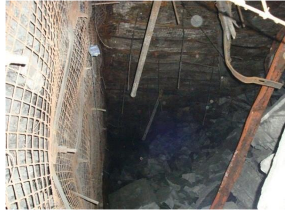
Fig. 5 Pillar deformation in 4301 working face goaf
