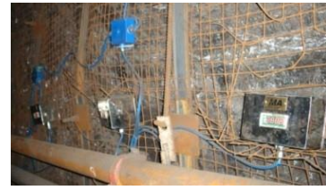
(a) Lateral deformation monitoring instrument
