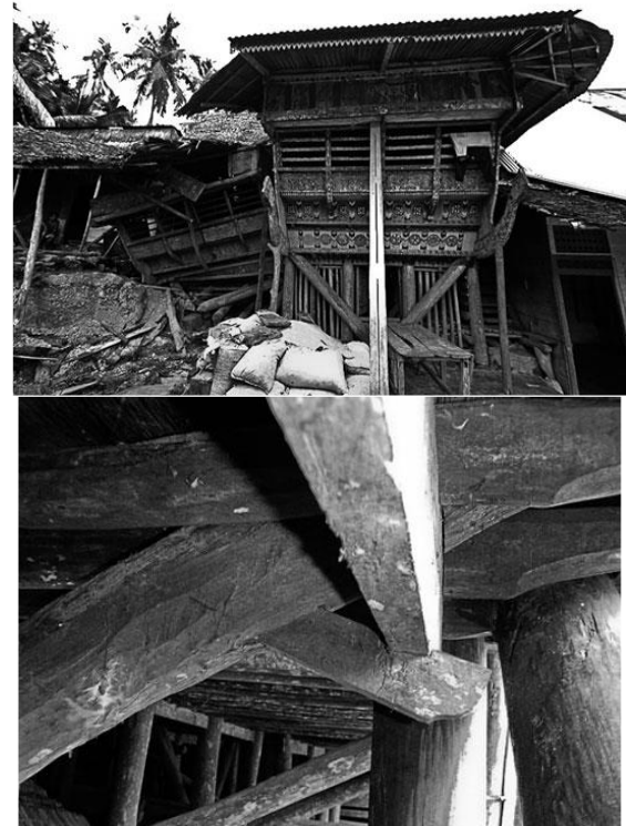
Fig. 8 Damaged Building B (Source: Solarino et al. 2017, Nitto et al. 2016)
