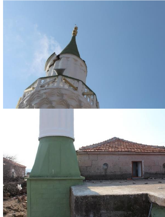
Fig. 11 Mosque and minaret damages
