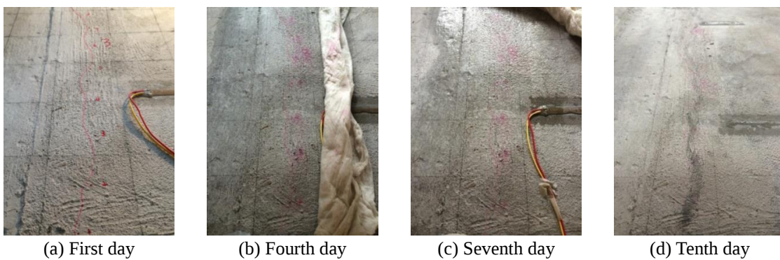
Fig. 15 Self-healing at the measurement points 3-1→3-16 for crack 3
