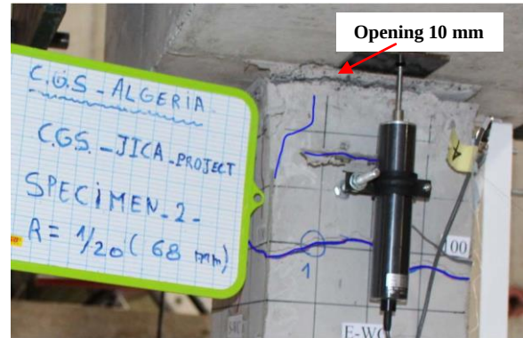
Fig. 23 Opening of 10 mm at top column-loading beam connection, 5% drift (specimen 2)
