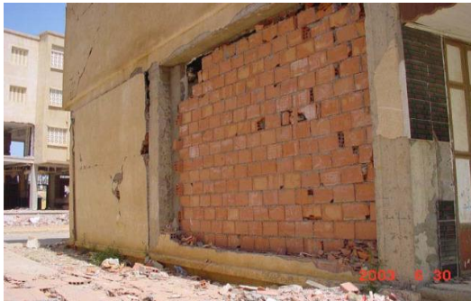
Fig. 2 Collapse of external infill walls of the first story
