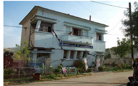
Fig. 4 General view of 2-story damaged masonry stone building
