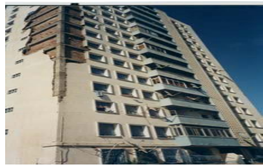
Fig. 3 Collapse of external infill walls of higher stories
