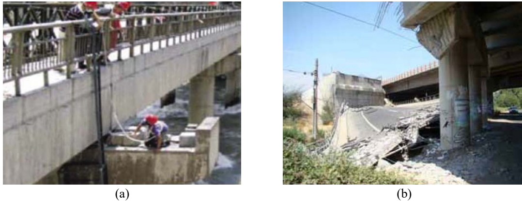
Fig. 1 Failures in seat-type skewed bridges: (a) 1.8 m transverse displacement in 80° skewed bridge, Mingjiang Bridge, China 2008 (Zhiqiang and Lee 2009); (b) Deck rotation from obtuse corner toward acute corner and span collapse in 40° skewed bridge (Yen et al. 2011b)
