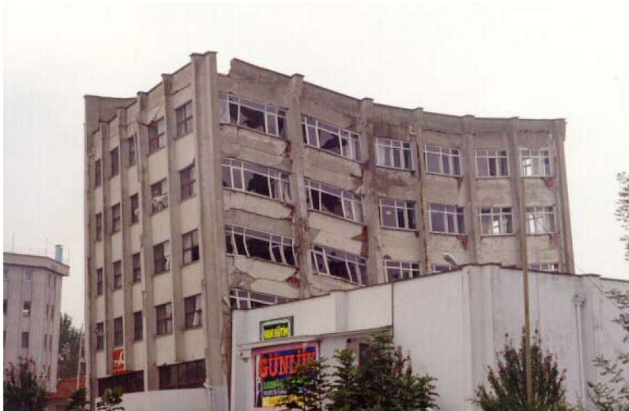
Fig. 4 A building heavily damaged during Marmara earthquake, Turkey in 1999 due to torsional irregularity
