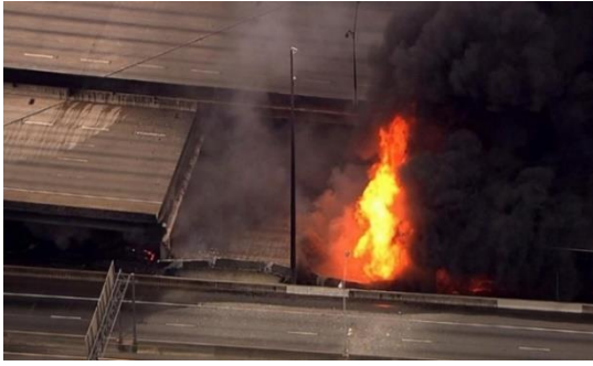
Fig. 2 Fire induced collapse of PC T shaped bridge girder in I-85 (Atlanta Chinese life network 2017, China.com - News Channel 2017, Huanqiu News 2017)
