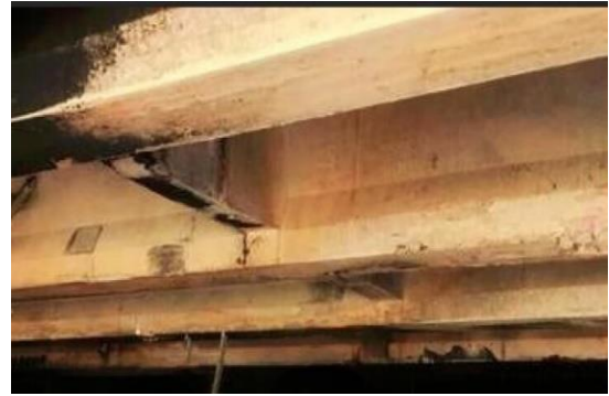
Fig. 3 Fire-damaged PC T shaped bridge girder (Maintenance online 2017)
