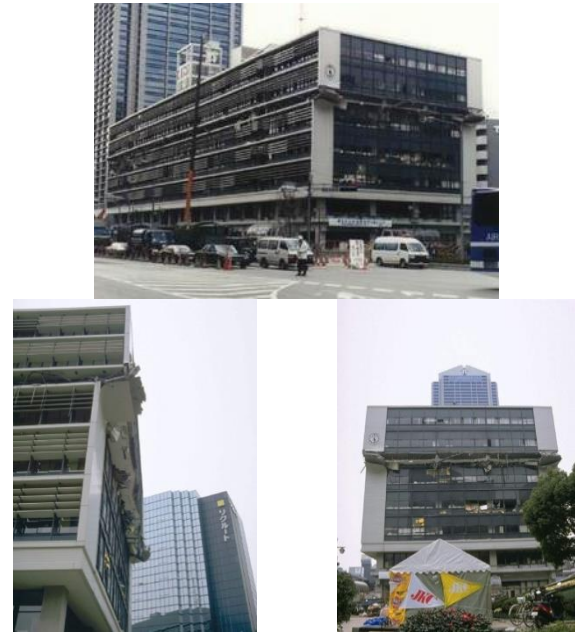
Fig. 2 Seismic damage of SRC-RC hybrid structures
